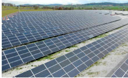
1 MW AZİZOĞLU INTEGRATED PLANT SOLAR POWER PLANT (SPP)
